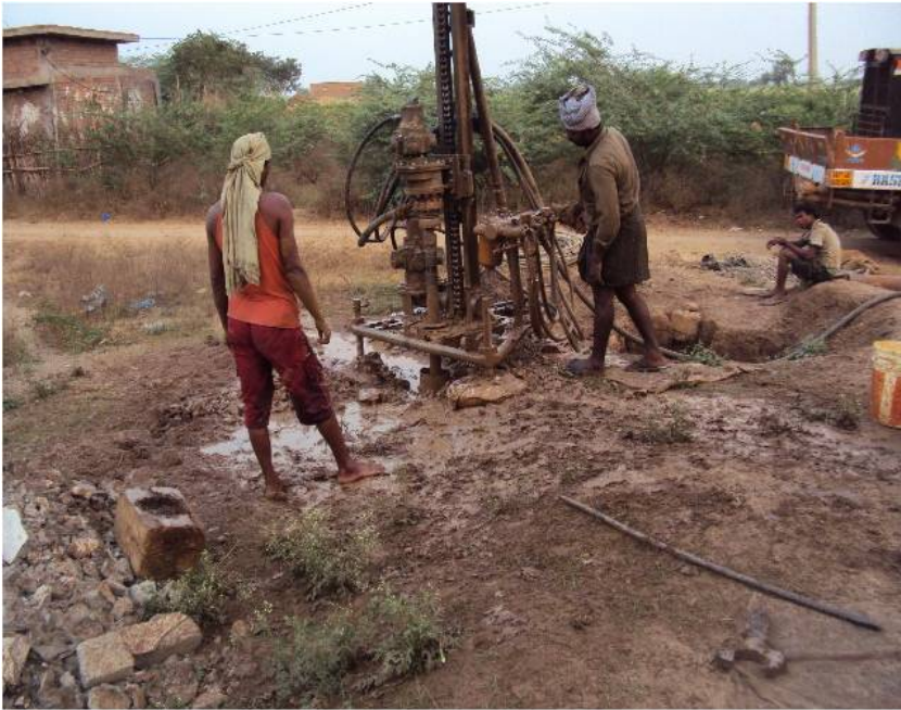
Project in Process and community residents assisting; taking ownership of the water project
